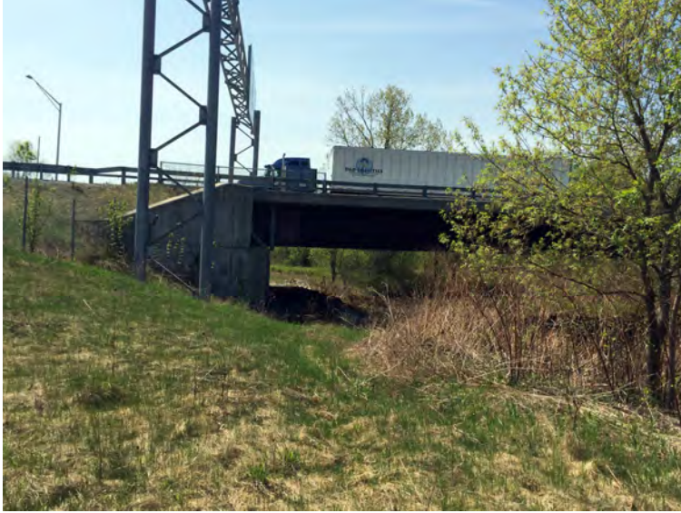
The Ninja Path will pass under VT-279. The over-pass was designed to accommodate a future path.
