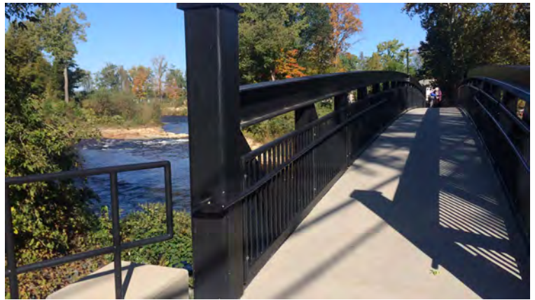
This bike/ped bridge spanning the Walloomsac River was replaced after Tropical Storm Irene and is a key connection between the Ninja Path and downtown Bennington.
