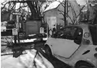
The Town of Bennington has installed several new high-speed electric vehicle charging stations in municipal parking lots in the downtown area.
